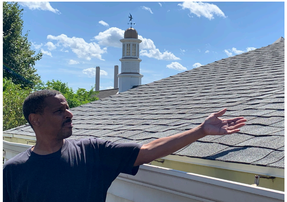
Forest Hudson shows the new gabled roof over the Delray Neighborhood House gymnasium.
